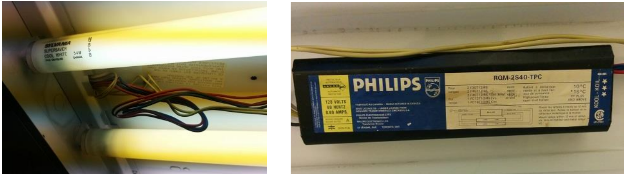
FIGURE 10. T12 FLUORESCENT LAMPS (LEFT) AND MAGNETIC BALLAST (RIGHT)
