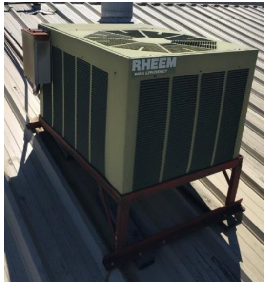
FIGURE 15. OLD ROOFTOP AIR CONDITIONER CONDENSER UNIT
