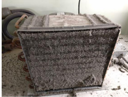
FIGURE 25. DEBRIS ACCUMULATION ON REFRIGERATOR CONDENSER
