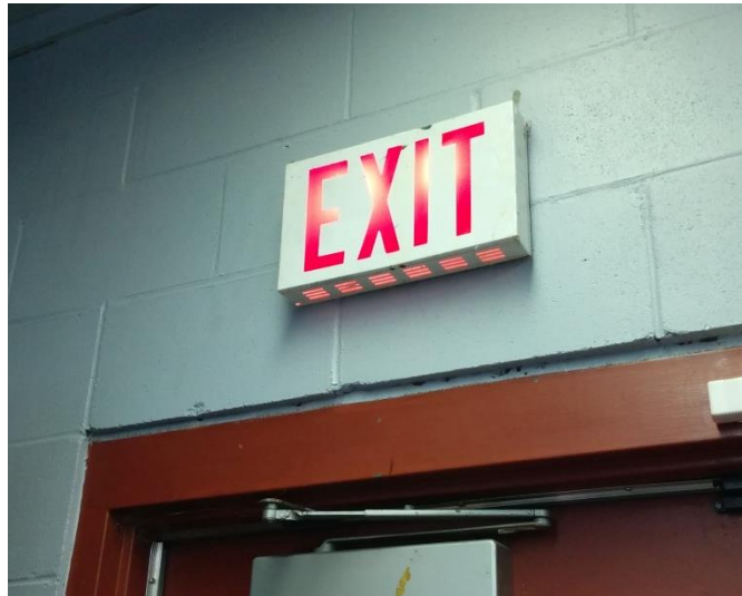
FIGURE 8. INCANDESCENT EXIT SIGN FIXTURE
